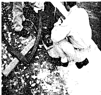
Photo.5 Valve of water
