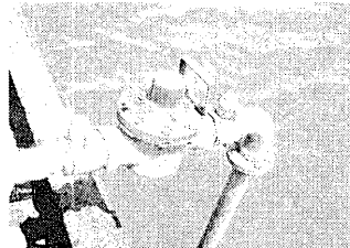
Photo. 5 Valve of water
