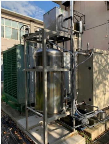
Fig. 21 Hot water pooling tank
