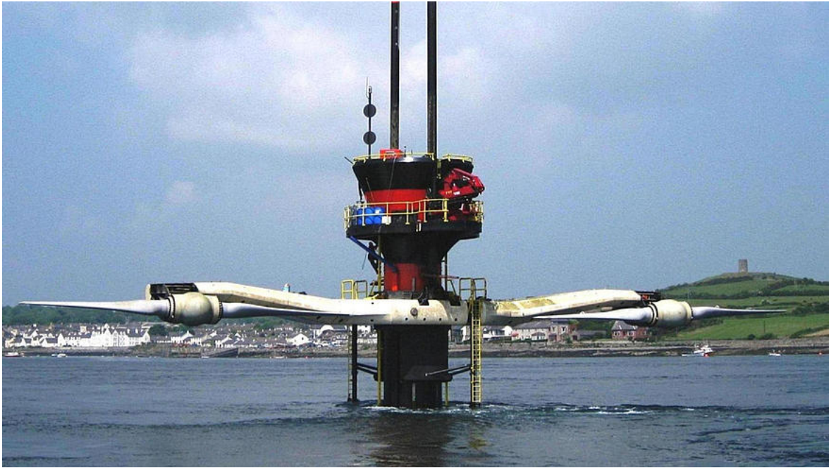
Figure 3-6. The SeaGen project in UK [© MCT].
